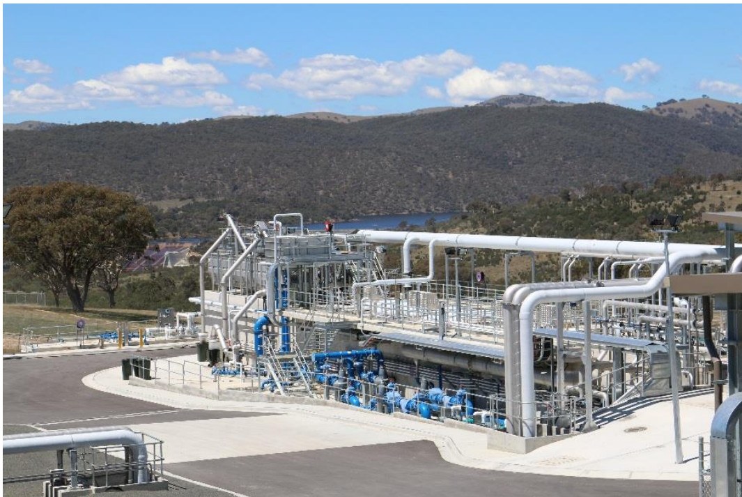
Figure 2: Membrane bioreactor at the Googong Water Recycling Plant
