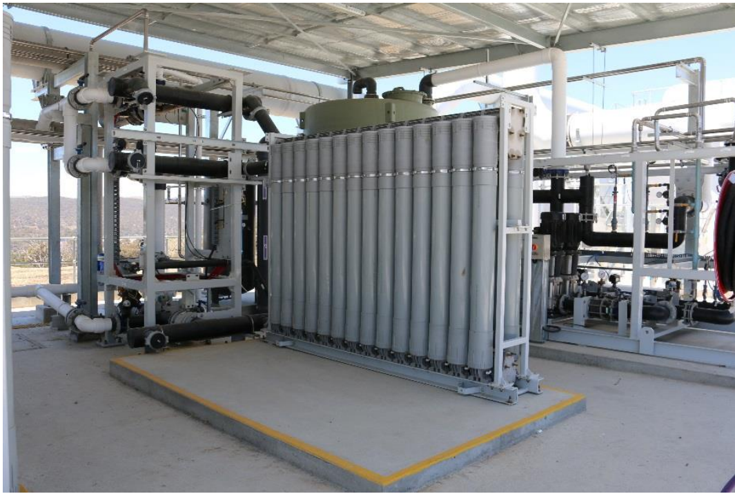
Figure 3: Tertiary filtration system at the Googong Water Recycling Plant
